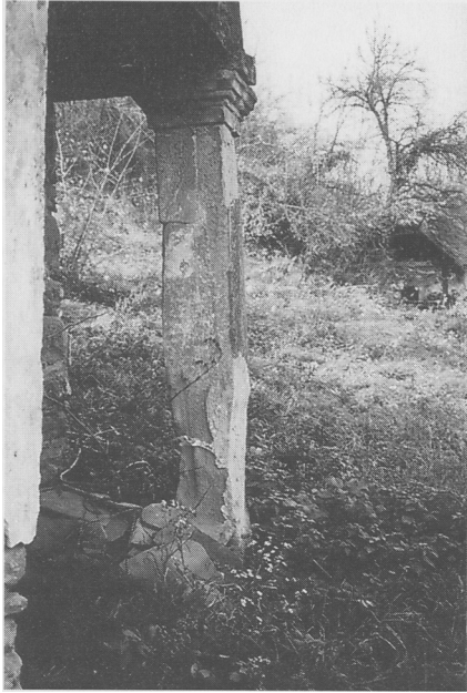
FIG. 3. Damaged stair pillar from the house used as the inn.
